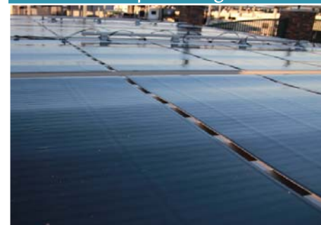
Solar Parking Canopies
