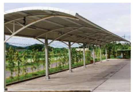
Solar Parking Canopies
