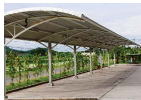
Solar Parking Canopies
